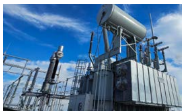
Onshore substation at Oneida in Jarvis, Ontario.
