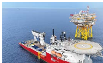
Hai Long offshore substation in the Taiwan Strait.
